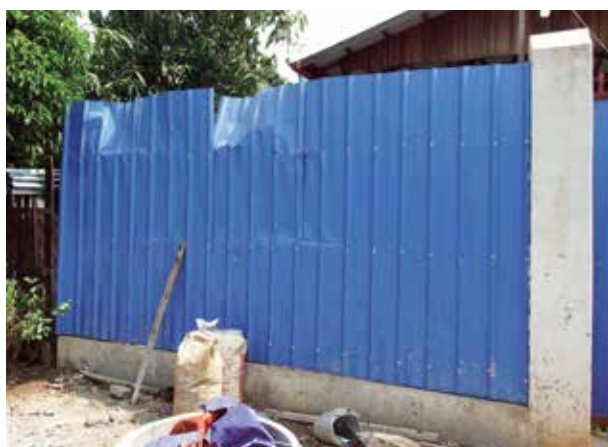
Damaged compound, Yesagyo. Photo: Rachel Fleming
